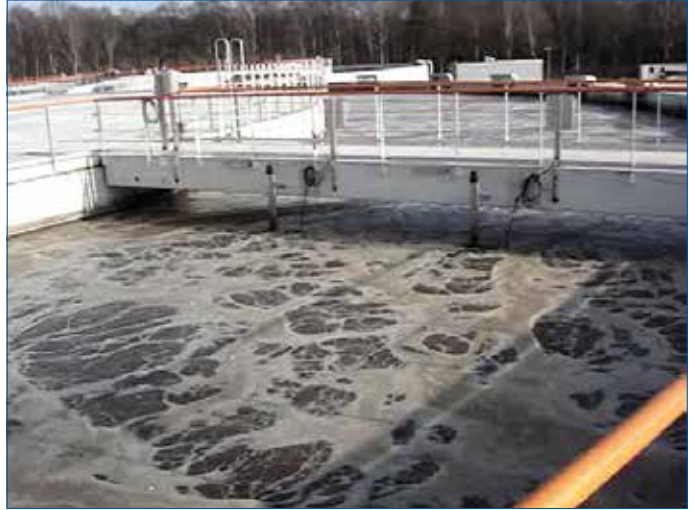
Fig. 19: Activated sludge tank
