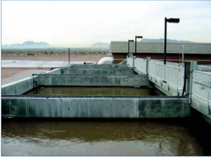
Fig. 12: Typical tank of a waste water treatment plant (Henderson, NV)
