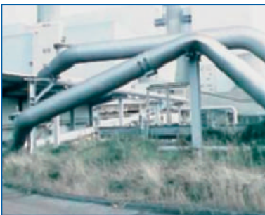
Fig. 1-a: Completely destroyed DN 600 discharge pipe (wall thickness 12 mm)
