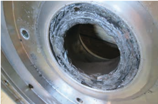
Broken bearing bush of process pump
