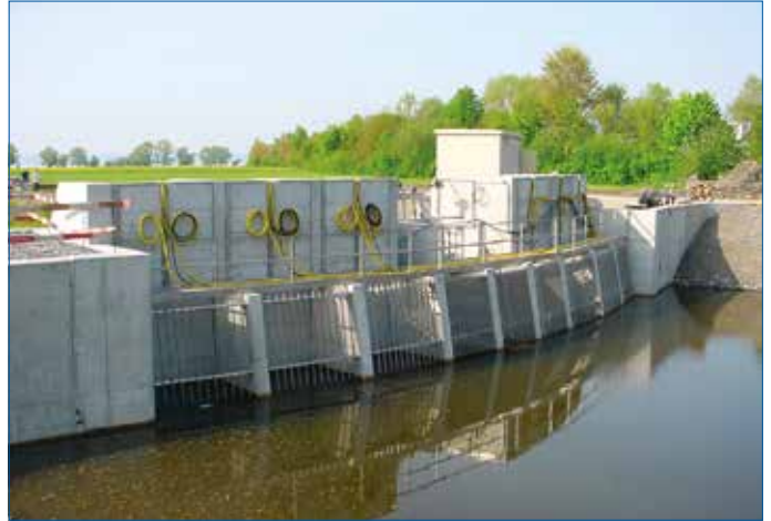
Fig. 65: Coarse screens upstream of an Amacan pumping station (water abstraction from a river)
