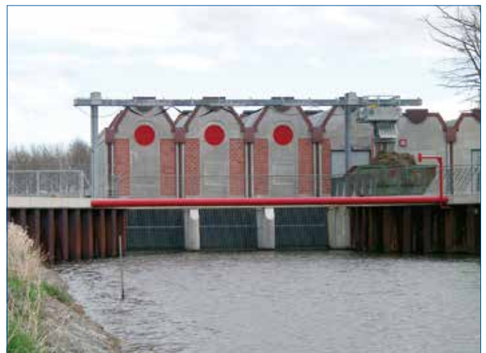
Fig. 73: Pumping station with automatic screens
