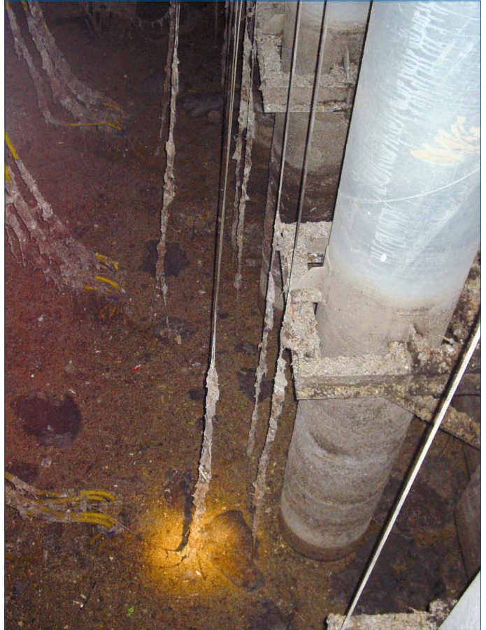
Fig. 91: Formation of a layer of scum in the pump sump
