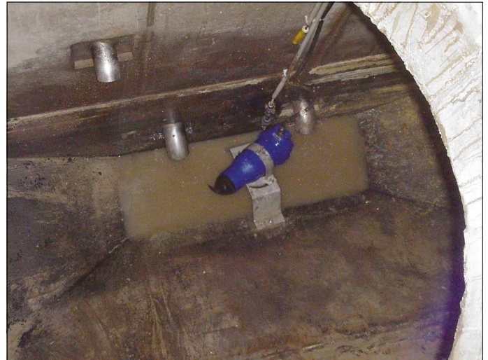
Fig. 102: Submersible motor mixer in the pump sump
