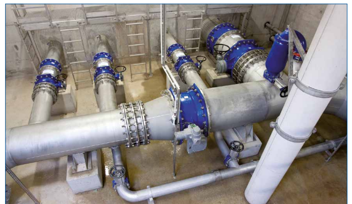
Fig. 54: Valve chamber with the piping integrated horizontally
