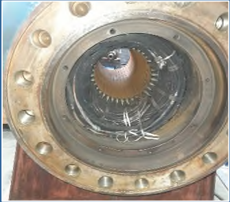
Existing damaged winding
