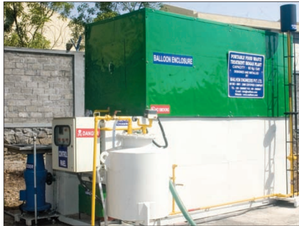
Installation of Bio-Gas Plant at Nashik plant - Generation of Bio-Gas with consumption of bio-waste.
