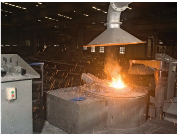
Fume extractor installed at Foundry division, Vambori
