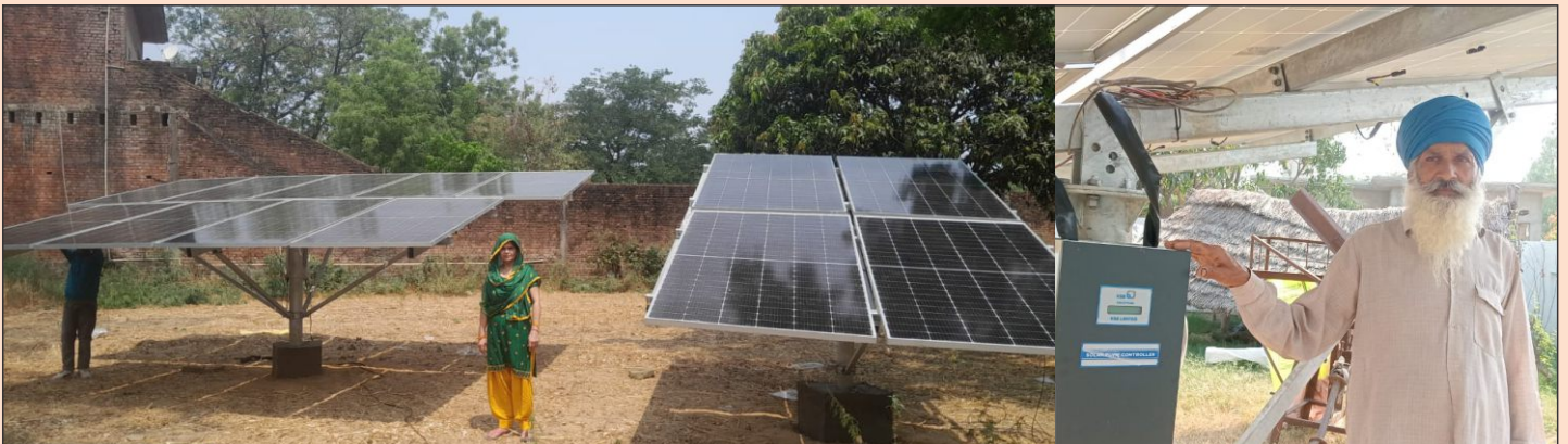
KSB Solar Pumping Systems installations at farms
