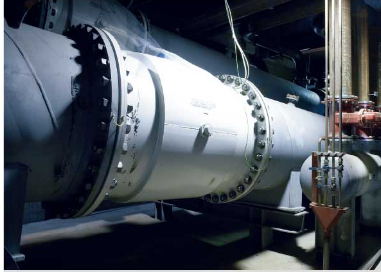
Test facility for cooling water pumps
