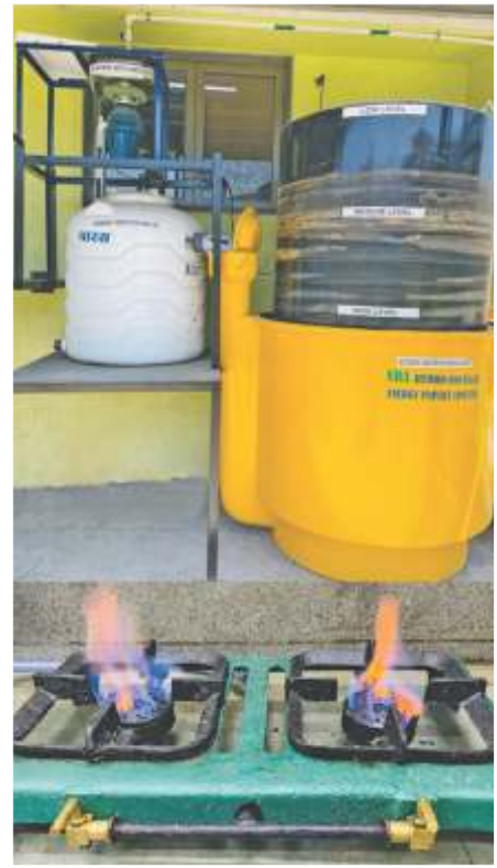
Biogas Plant at Shirwal
