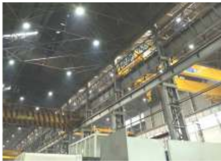
LED Bulb in offices and shop floor
