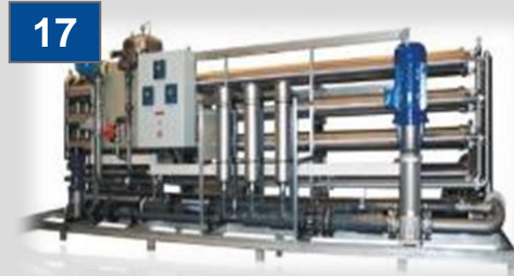
Filtration Plant System: (RO & UF)
