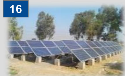
Solar Pumping System
