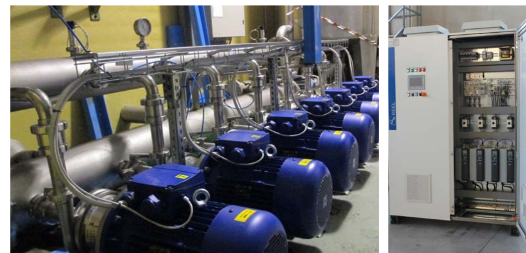
Command and control panels and SuPremE motors in a pumping plant at a mineral water production factory
