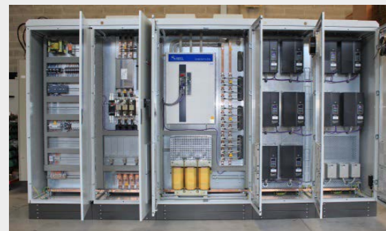
Command and control panel for a CHP plant.
