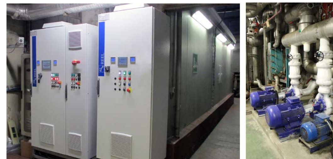
Deaerator circuit command and control panels and pumping system equipped with SuPremE motors for the glycol cooling circuit at the Galbani factory
