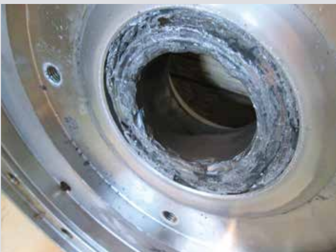
Broken bearing bush of process pump
